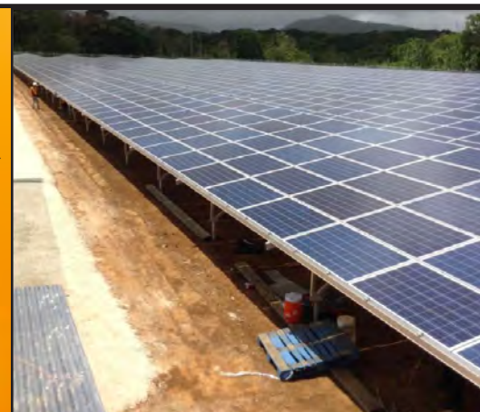
600kW solar farm at Pohlenghas Madolenihmw
