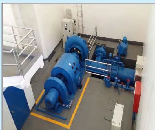
Nanpil Hydro plant 725kW
