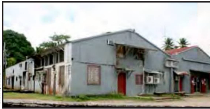
PUC's "luxurious" Administration Building in downtown Kolonia. The building's sign above the door long ago disappeared and at least one of the walls has collapsed.
