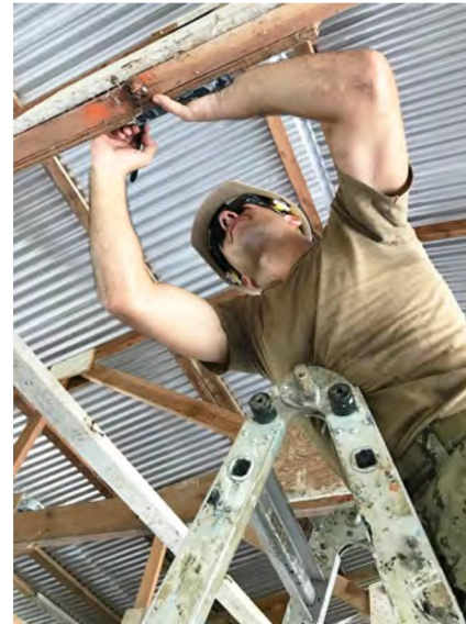
KOSRAE, Federated States of Micronesia (March 29, 2017) Construction Electrician 3rd Class Edwardo Blanco, from Atlanta, Georgia, marks where trusses of the elementary school need to be cut to renovate the ceiling on the Naval Mobile Construction Battalion (NMCB) 1 elementary school project in Malem on Kosrae, Federated States of Micronesia, March 29, 2017. NMCB 1 is forward deployed to execute construction, humanitarian and foreign assistance, special operations combat service support, and theater security cooperation in support of U.S. Pacific Command. (U.S. Navy photo by Utilitiesman Constructionman Matthew Konopka)
