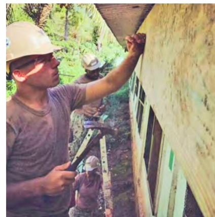
KOSRAE, Federated States of Micronesia (May 9, 2017) Construction Electrician 3rd Class Eduardo Blanco, from Atlanta, Georgia, nails in formwork for the Naval Mobile Construction Battalion (NMCB) 1 Elementary School in Malem on the island of Kosrae, Federated States of Micronesia, May 11, 2017. NMCB 1 is forward deployed to execute construction, humanitarian and foreign assistance, special operations combat service support, and theater security cooperation in support of U.S. Pacific Command. (U.S. Navy Photo by Utilitiesman Constructionman Matthew Konopka)
