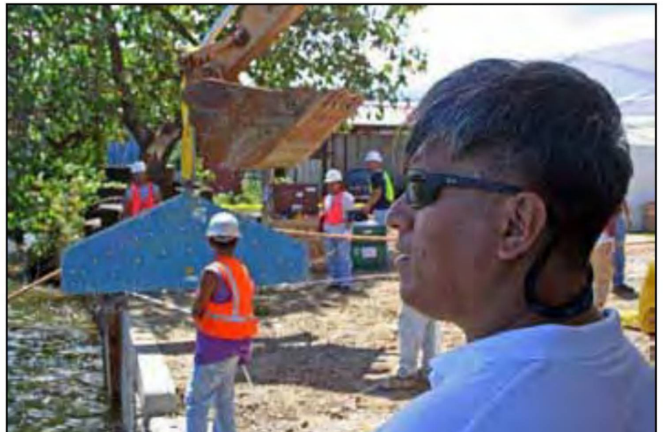
Telecom Customer Care Officer Fredy Perman watches as the cable is pulled to shore
