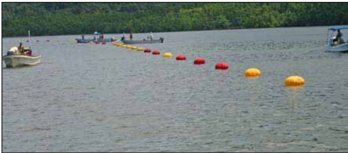
Locally hired boat crews work to move the cable into its final position before cutting the inflatable buoys and sinking the cable
