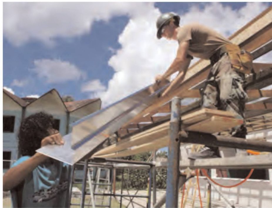
Marvin Mino helps Steel Worker 3rd Class Michael Featherston with a gutter at Mwan Elementary School in Chuuk - Photo by Mass Communication Specialist 2nd Class (SW/AW) James Seward and a garden hose.
