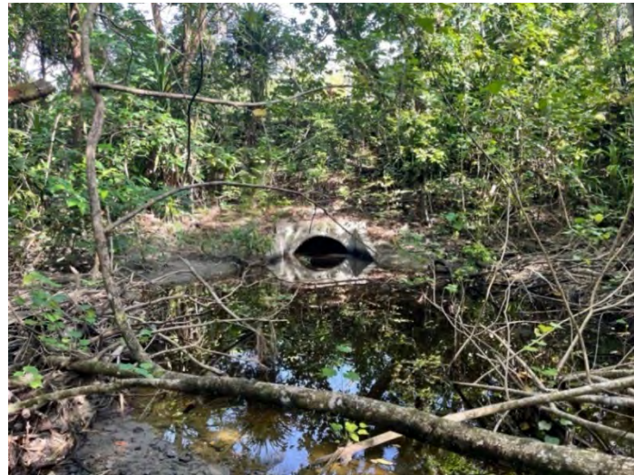
Photo 30. Culvert located south of airport near main road on the edge of the Galil mangrove.
