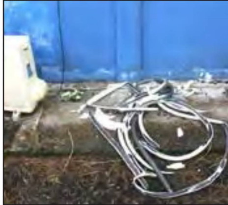
Thieves stripped the insulation from Freon tubes and left it next to this pillaged air conditioner Nigel Jaynes - The Kaselehlle Press
