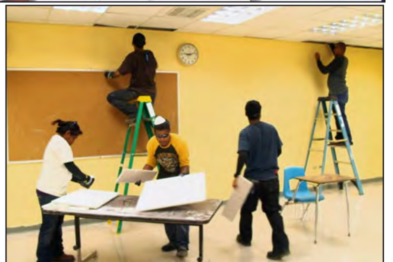
Repairing classrooms at Southern High School under GDOE’s Facilities Work Training Program
