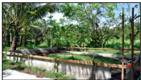
Setting the foundation works for the dry litter piggery model in Nanpil Nett
