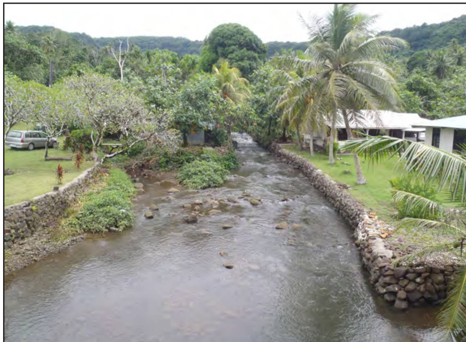
Stone walls lining the river at Alamoar Church on Pohnpei are probably modern counterparts of much older structures intended to stabilize the river banks and even to reclaim land along this narrow coastal strip. Photo by Patrick Nunn.
