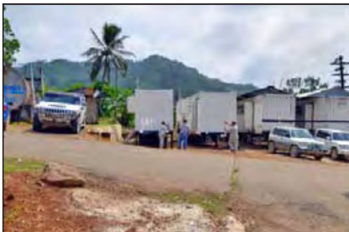
Governor Johnson Elimo starts one of the new generators – "That feels very good!" was his comment as the generators hummed into life
