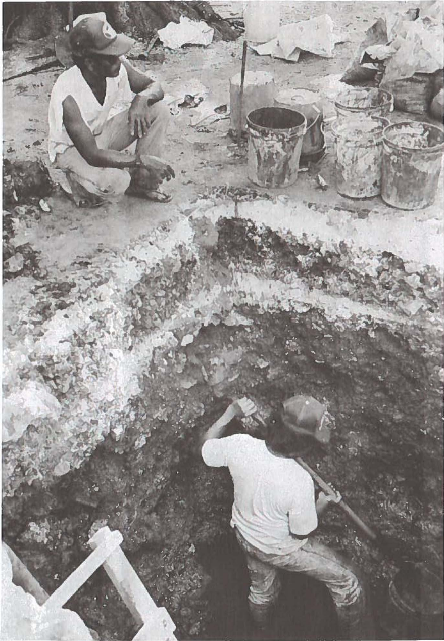
Figure 3. Excavation of submerged pottery deposits below islet fill in Katem compound of Lelu Island. Nena Lonno is excavating while Kerick Benjamin is waiting to haul up buckets of sediment for water-screening.
