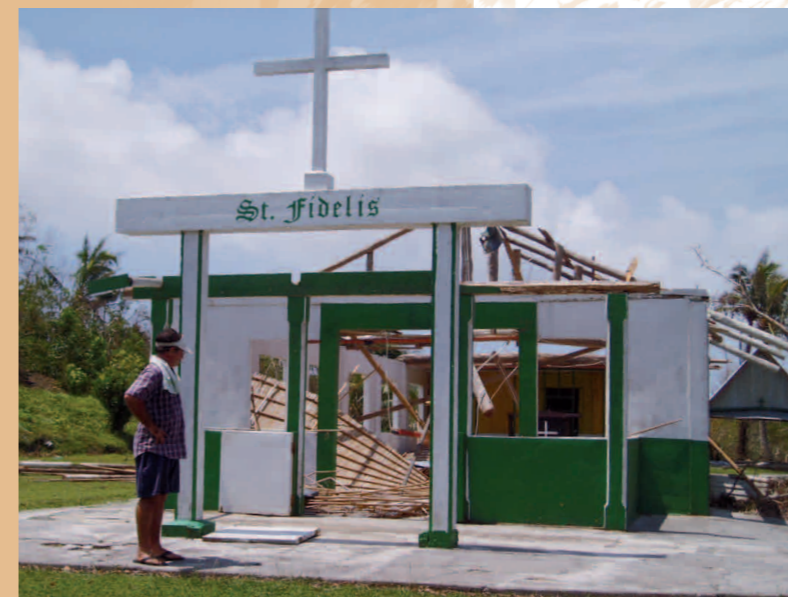
St. Fidelis church in Kanif with typhoon damage, 2006
