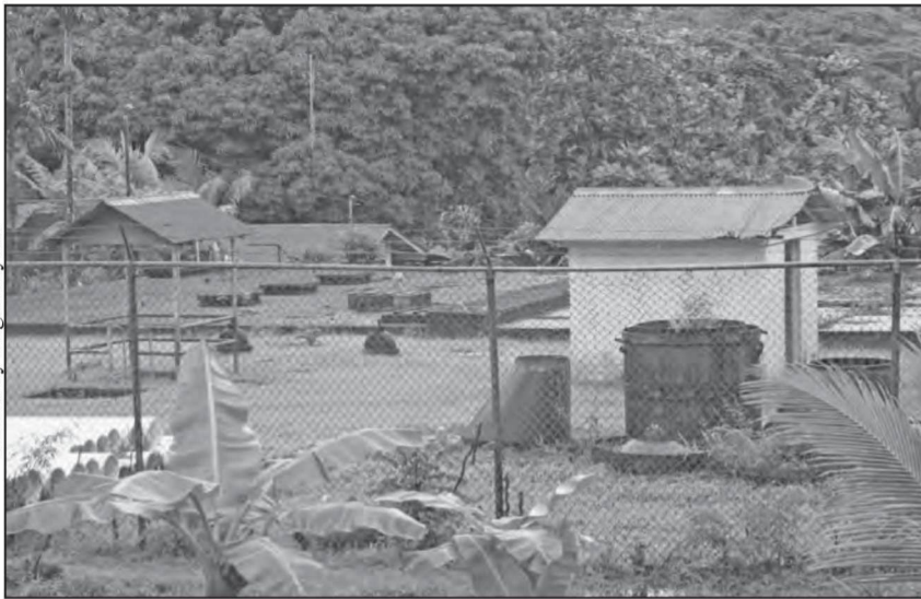
PUC water treatment plant in Nanpohnmal, Pohnpei
