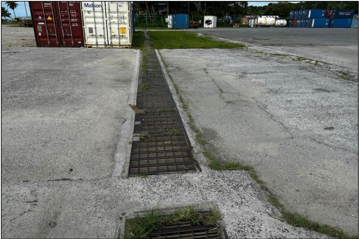
Photo 11: Storm drain channel which encircles the gated area within the port and leads toward the ocean. Photo is looking south.
