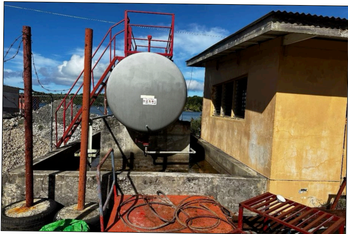
Photo 16: Overview of 10,000-liter diesel AST located at the YFA facility. Note: A concrete containment basin sits beneath the AST. Photo is looking south.
