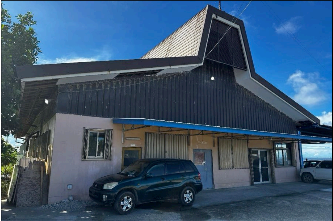
Photo 17: Overview of the office building at the YFA premises. Photo is looking east.
