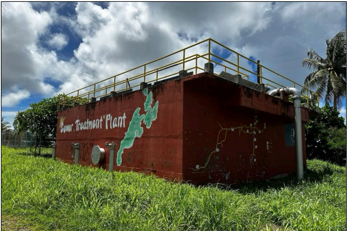
Photo 20: Overview of wastewater treatment plant located near the eastern boundary of the subject site. Photo is looking east.
