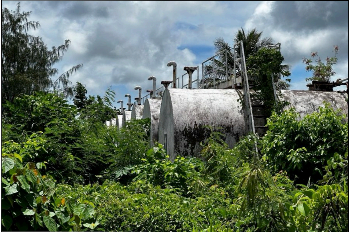
Photo 23: Zoomed-in photograph of the seven abandoned former U.S. Coast Guard fuel tanks. Photo is looking southeast.
