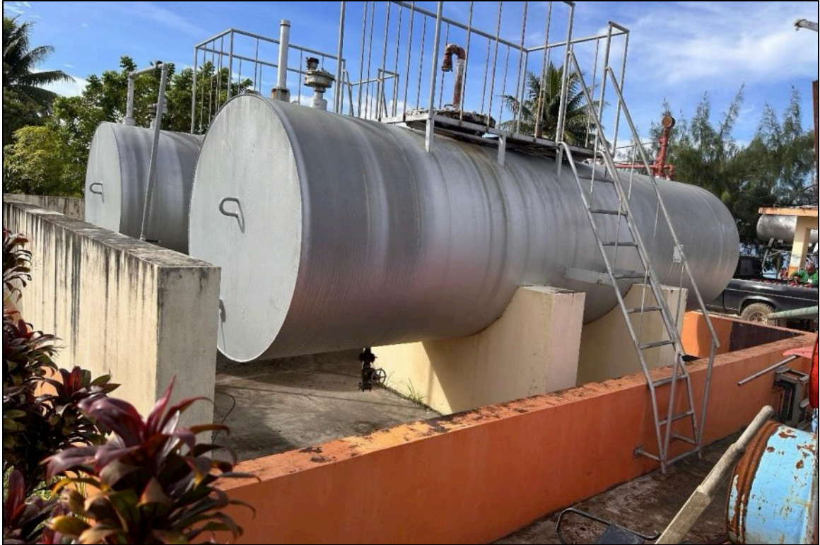
Photo 27: Overview of two steel ASTs containing diesel (3,700 gallons) and unleaded gasoline (4,010 gallons) in a concrete secondary containment observed at YCA Rufan Gas Station. Photo is looking north.
