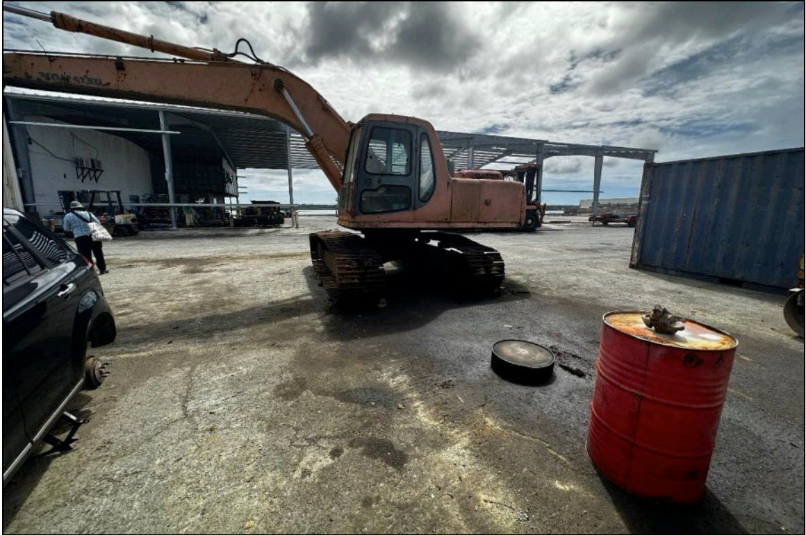
Photo 7: Closer look at other area within the main port maintenance shop displaying concrete staining. Photo is looking northeast.
