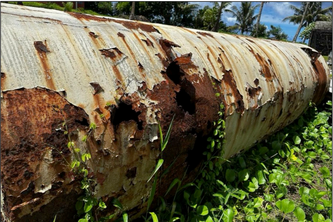
Photo 22: Close-up view of empty, deteriorated AST observed adjacent to the abandoned vehicle piles. Photo is looking west.
