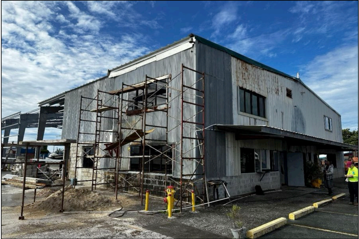
Photo 13: Overview of the front side of the Waab Transportation Company structure used as an office. The rear end is used as a warehouse. The building was under renovation during site visit. Photo is looking south.
