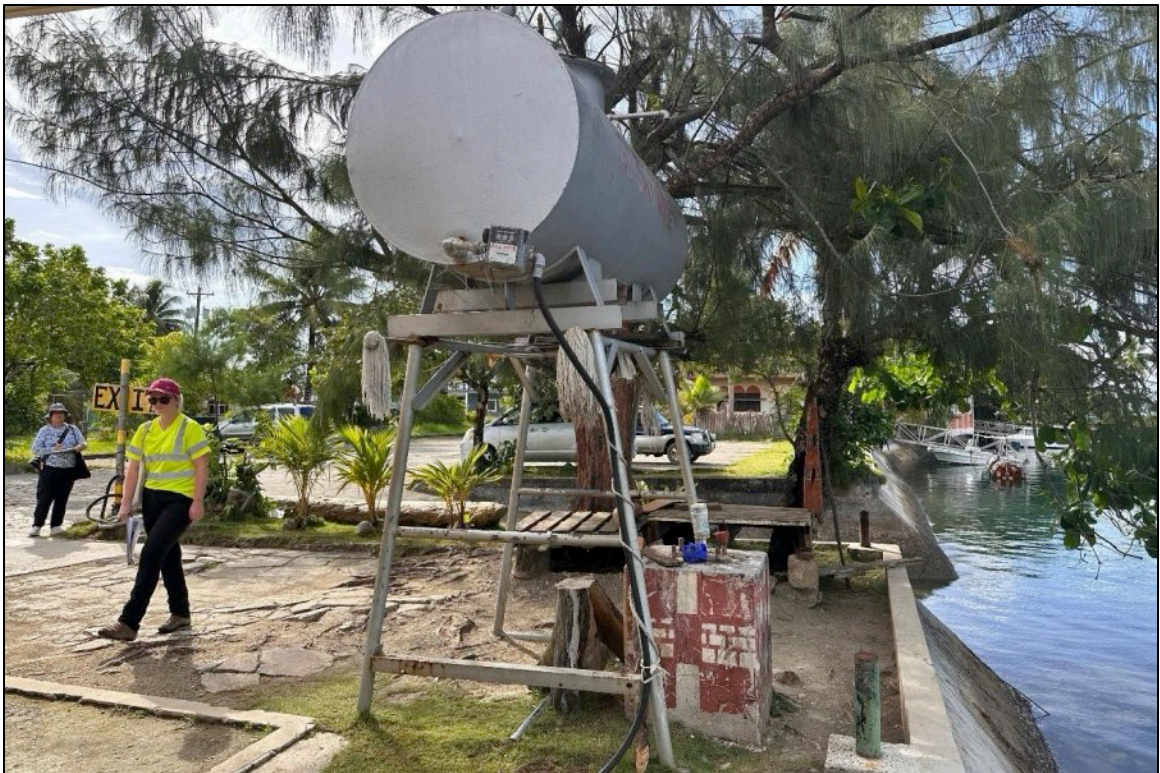
Photo 28: Overview of 320-gallon kerosene AST lacking secondary containment. Photo is looking east.
