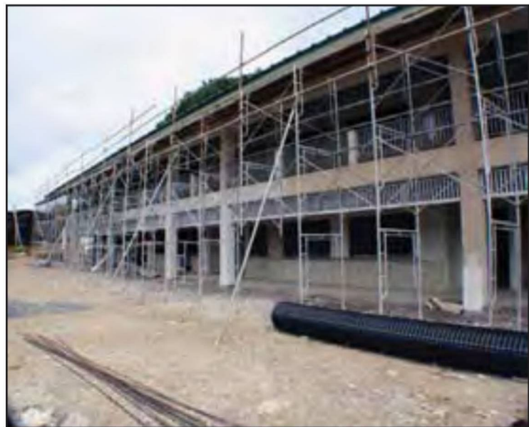
Nearly completed Kolonia Elementary school classroom being built by VCS Construction without a performance bond
