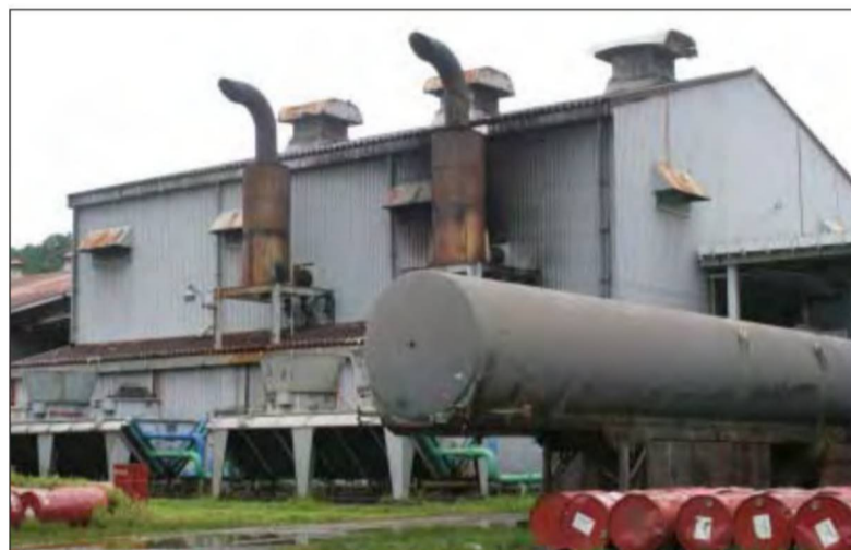
Pohnpei Utilities Company Power Plant in Nanpohnmal, Pohnpei
