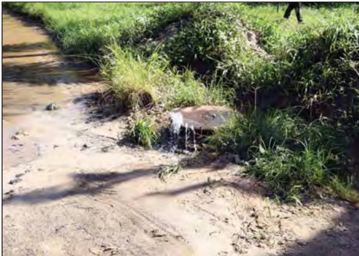
This photo of overflowing sewer pipes was taken in Chuuk three years ago
