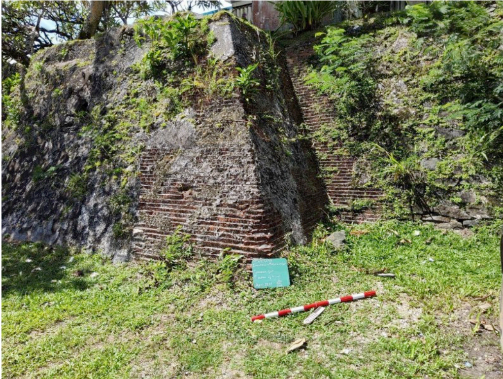
Figure 3-17 Feature 06, Northeast Corner Built of Coursed, Mortared Brick; View Facing Southeast; Note the Remnant Plaster
