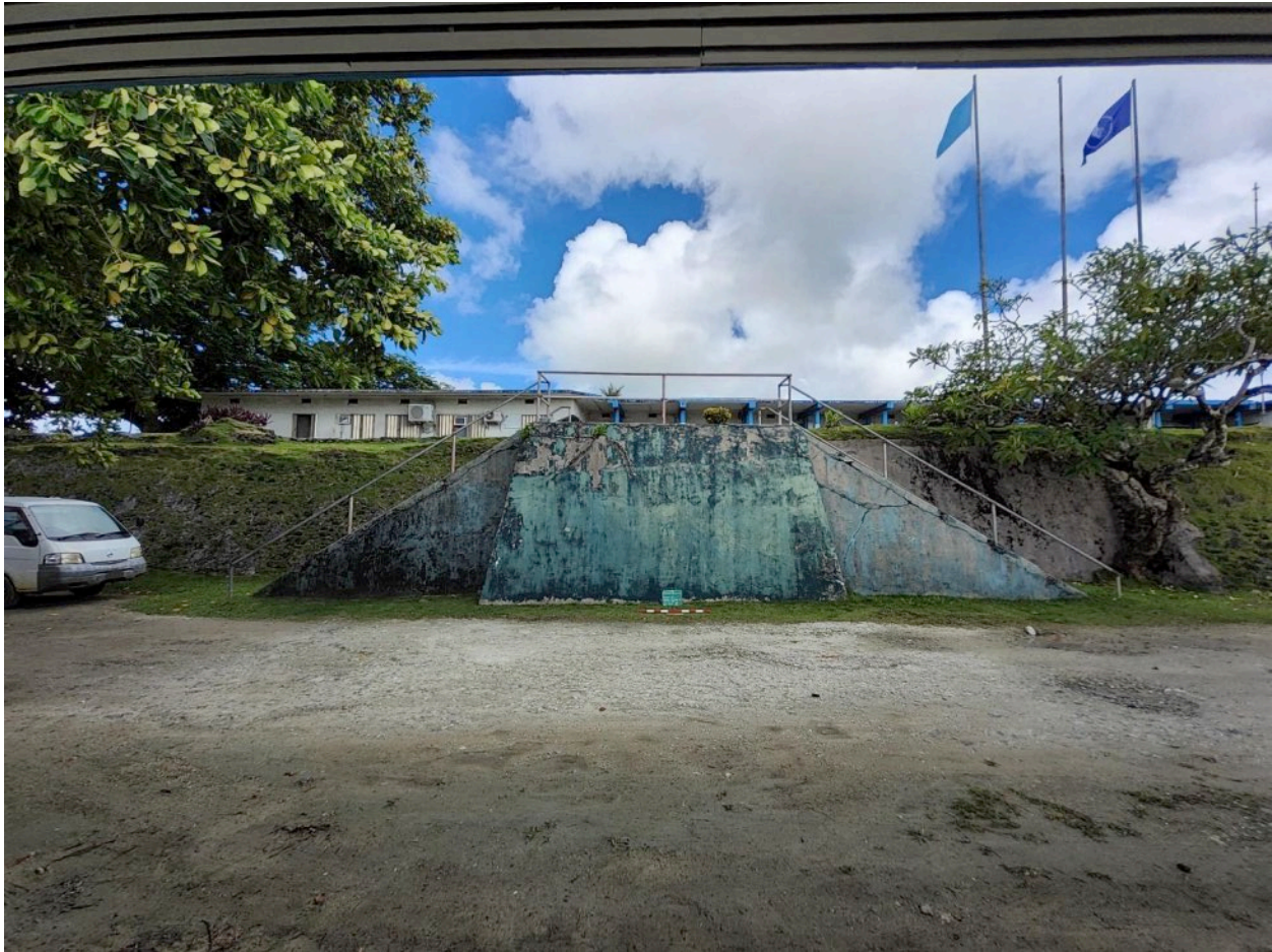
Figure 3-4 Feature 01 Overview, a Pair of Large Concrete Staircases Built along the East Side of the Spanish Fort during the Japanese Administration; View West; Staircases Built against Feature 06, the Spanish Colonial Earthen and Masonry Embankment
