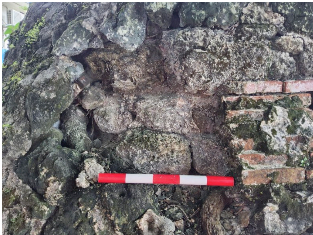
Figure 3-16 Feature 06, Detail of the Southeast Corner Showing Rubble (Left), Rough Ashlar (Center), and Brick (Right) Construction; View North
