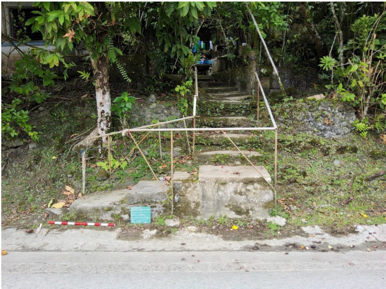
Figure 3-27 Temporary Site 01, Stone and Coral Retaining Wall with Japanese-era Concrete Steps, in Woorwoo Village, Rull Municipality; View South
