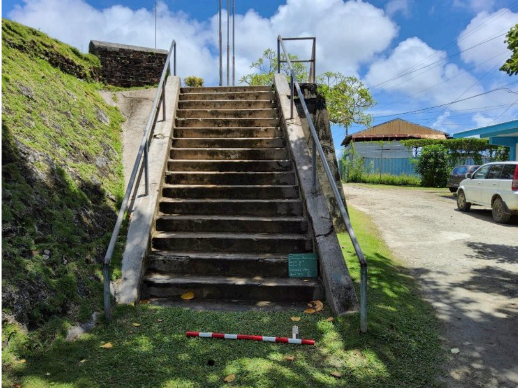
Figure 3-5 Feature 01, Close-up of One Flight of the Japanese Administration Stairs on the East Side of the Site; View North
