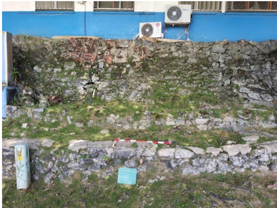
Figure 3-22 Feature 06, Section of the South Wall Damaged and Rebuilt Using Original Spanish Brickwork Fragments; View North
