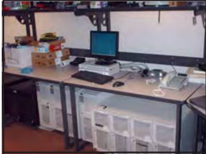
A few of the 30 servers that handle Telecom's internet service
